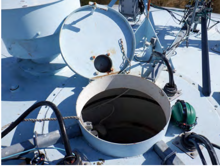
25) The access tube manway is in good condition. There is a four inch vent attached to the manway cover.
