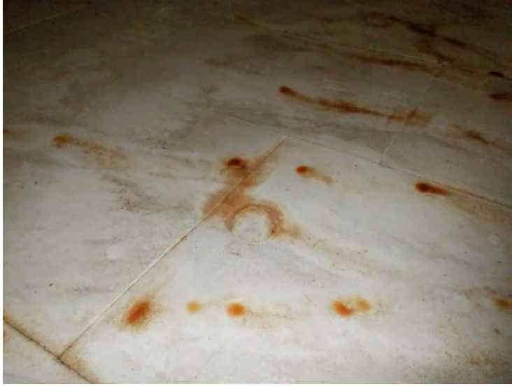
37) Spot coating failures to the substrate on the condensate platform.
