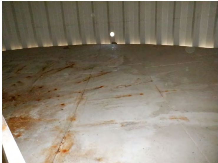
35) The coating on the condensate platform is in poor condition.
