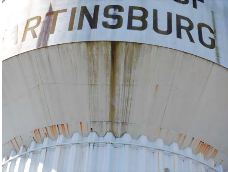
10) There are numerous coating failures to the substrate on the bowl.
