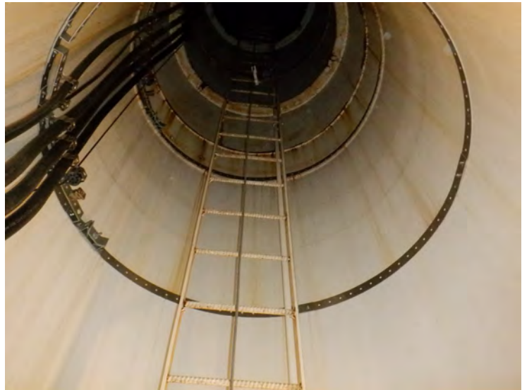
44) The coating in the access tube is in poor condition overall.
