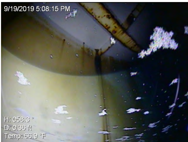
54) Edge corrosion on the roof painter's rings.
