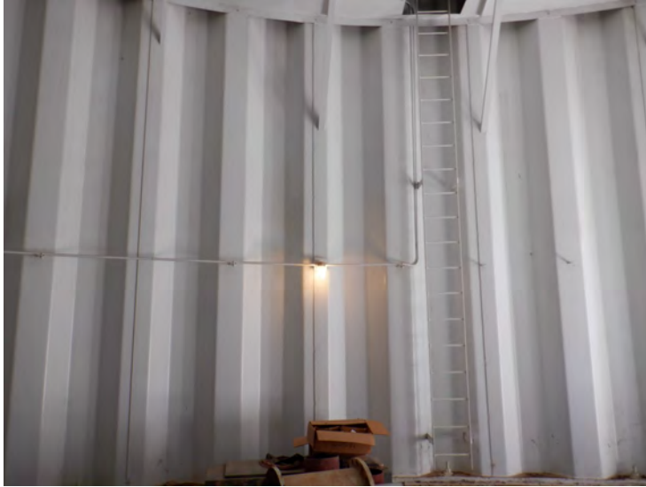
31) The lights were functioning during the inspection.
