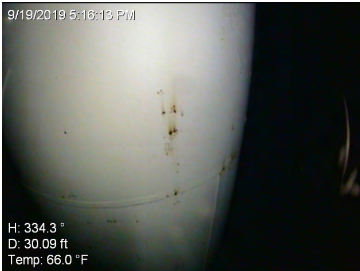
73) Spot coating failures to the substrate on the access tube.
