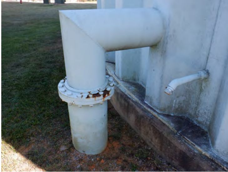
4) The overflow pipe elbows downward and routes directly underground.
