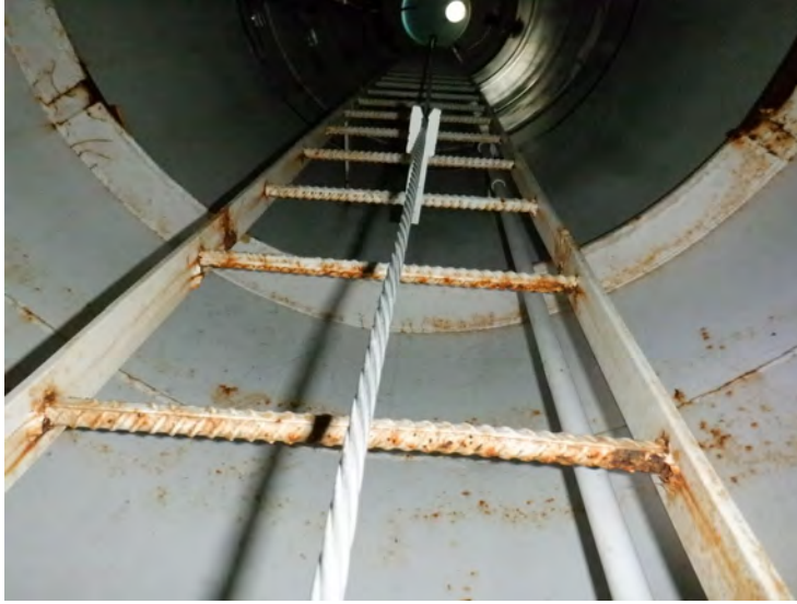
46) Spot coating failures to the substrate on the access tube ladder.
