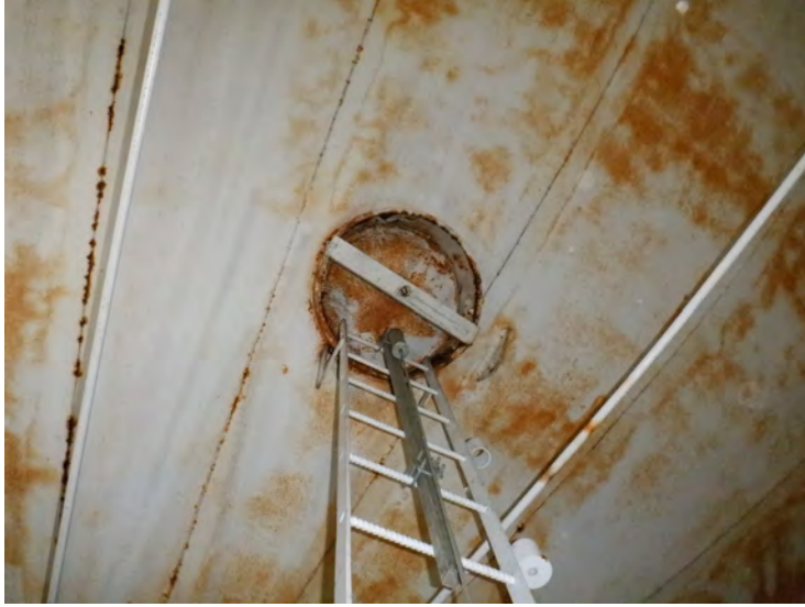
40) The bowl manway coating is in poor condition.
