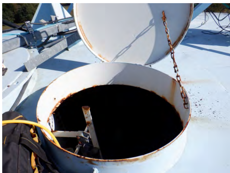
27) The wet interior roof hatch coating is in poor condition.
