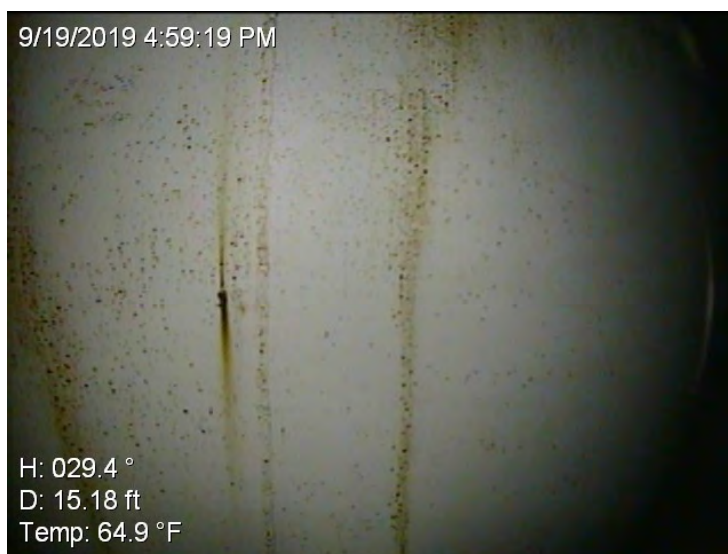
62) Pinhole coating failures on the sidewall.
