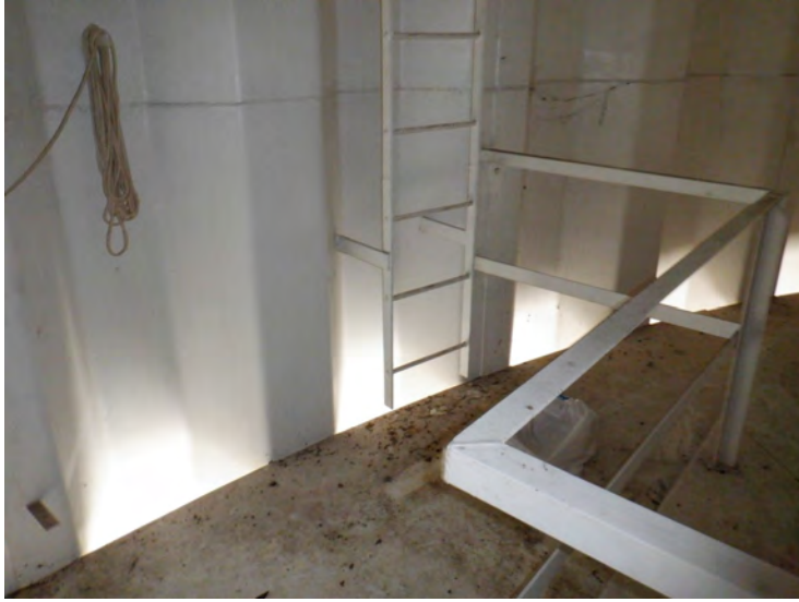
34) The ladder leading to the bird hatch does not have a fall prevention device.
