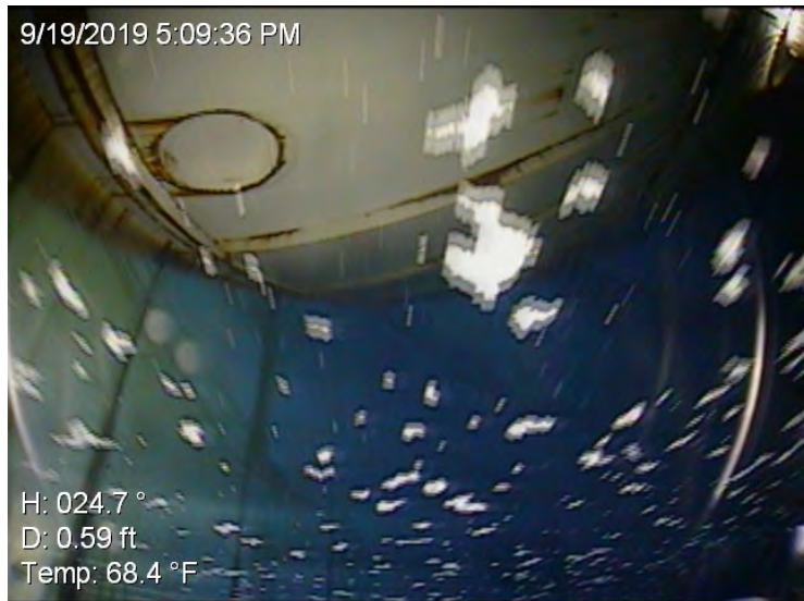
53) Weld burns and spot coating failures to the substrate on the wet interior roof panels.
