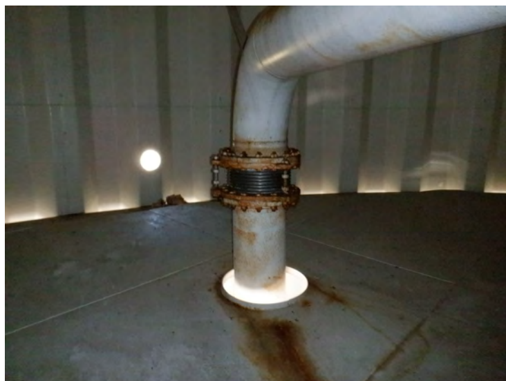
39) The expansion joint on the fill pipe is in good condition. There are spot coating failures on the flanges and hardware.
