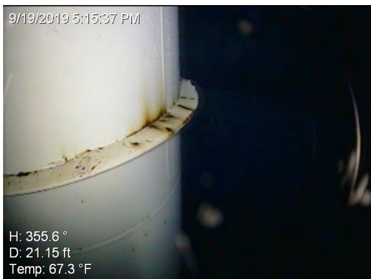
72) Spot coating failures to the substrate on an access tube stiffener.
