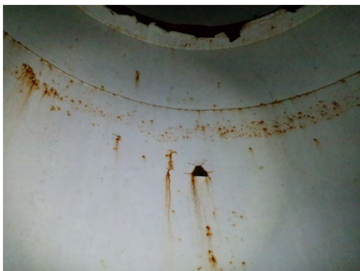
48) There are numerous spot coating failures to the substrate inside the access tube.
