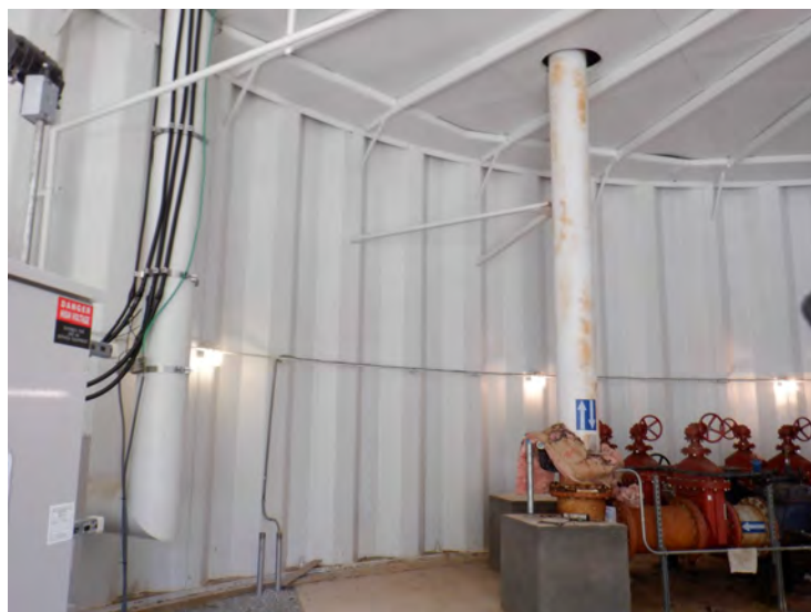
30) There is rust bleedthrough on the fill pipe throughout the dry interior.
