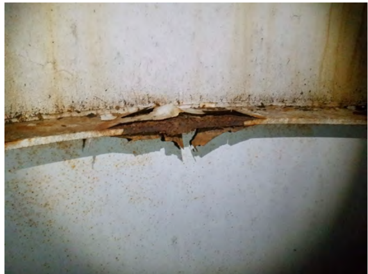
47) There are spot coating failures with rust undercutting on the access tube stiffeners.
