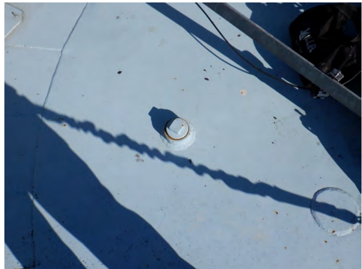
26) There is minor corrosion on the roof coupling threads.
