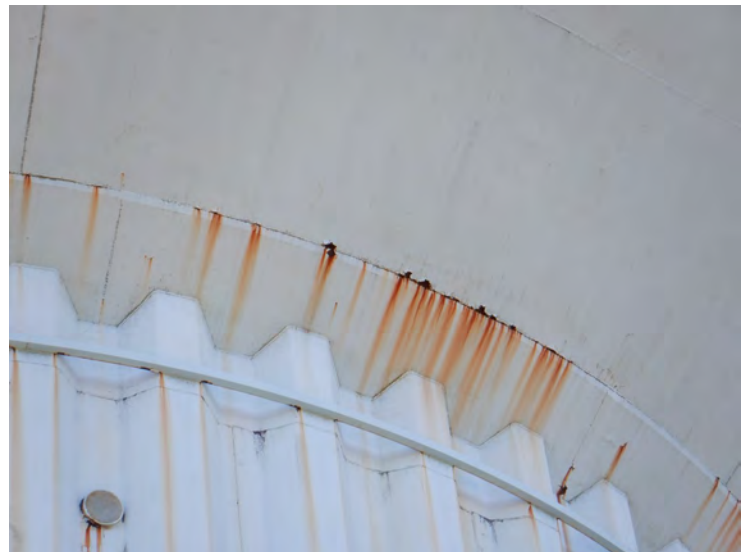
11) Spot coating failures with rust undercutting on the bowl.
