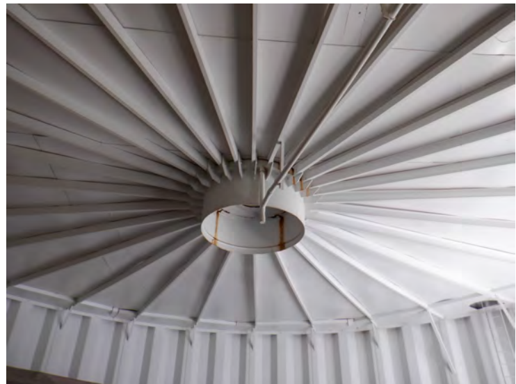
32) The coating on the underside of the condensate platform is in good condition.
