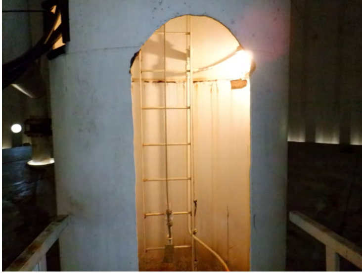
43) The access tube ladder is equipped with a cable style fall prevention device.
