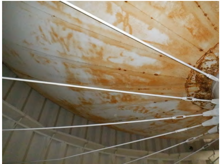
41) There is rust bleedthrough throughout the bowl.
