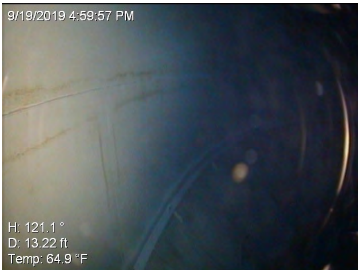
61) The sidewall coating is in fair condition.
