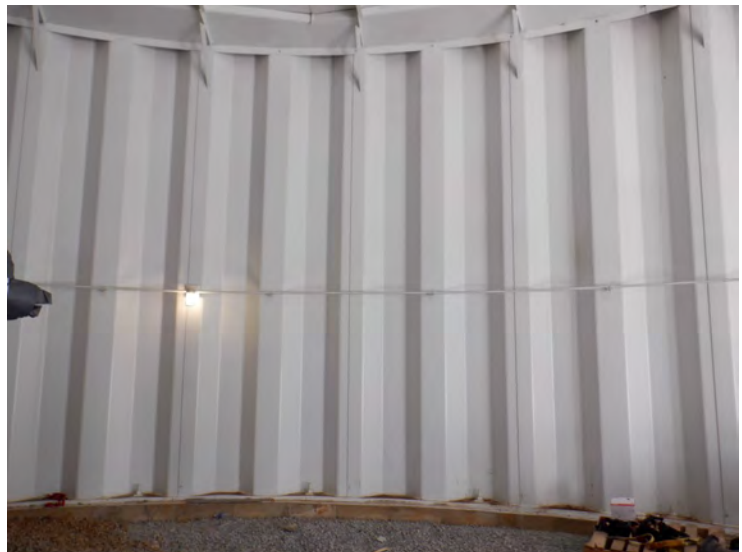
29) The coating on the column below the condensate platform is in good condition.
