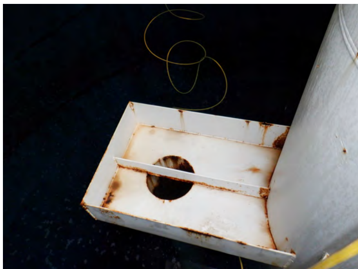
69) There are numerous spot coating failures on the overflow weir box.
