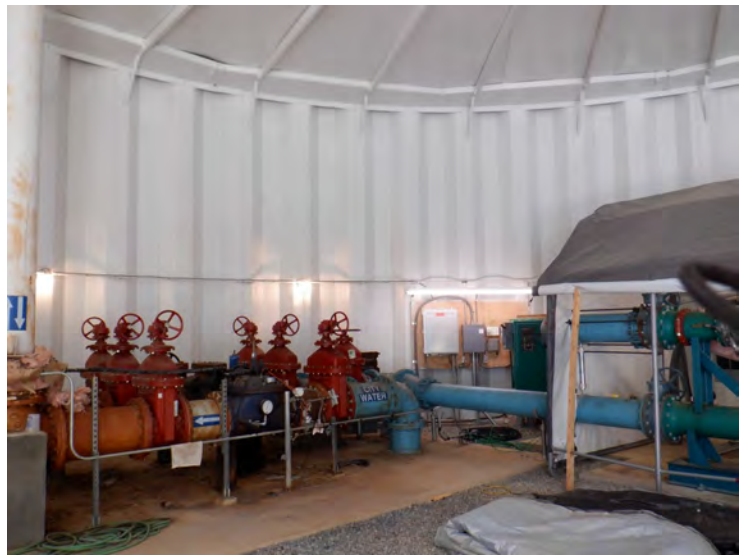
86) The coating on the piping above the floor in the column is in fair to poor condition.
