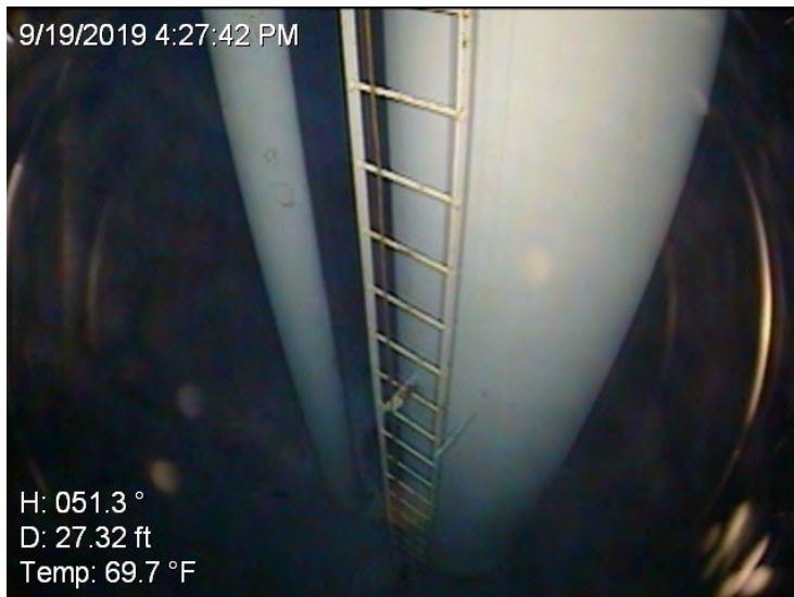
70) The wet interior ladder is equipped with a cable-type fall prevention device.
