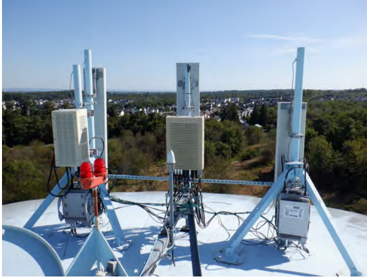
19) Roof antennas are mounted to tripods bolted to the roof.
