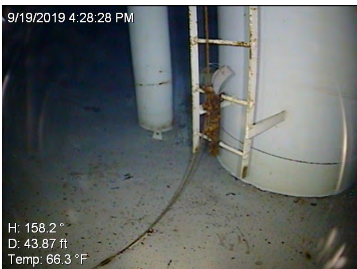
75) There is some corrosion on the bottom fall prevention ladder bracket.
