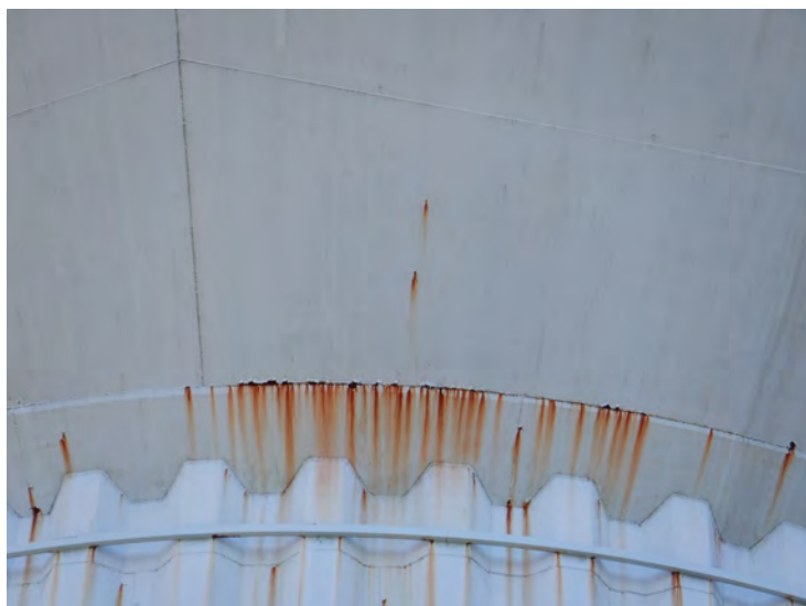
12) Coating failures are on both the weld seams and randomly throughout the flat panels.
