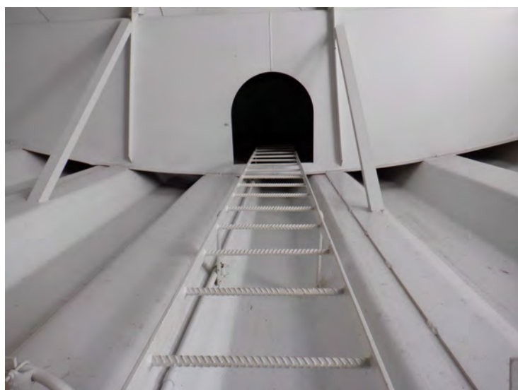
33) The column ladder is in good condition, but does not have a fall prevention device.
