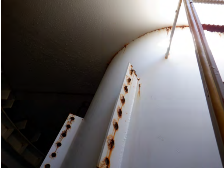
67) Spot coating failures to the substrate at the top of the access tube above high-water line.
