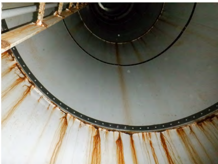
45) There are spot coating failures behind an expansion bracket inside the access tube.
