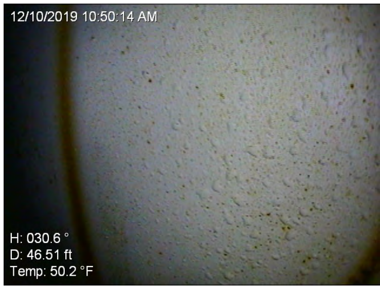
28) Coating blisters on the sidewall.
