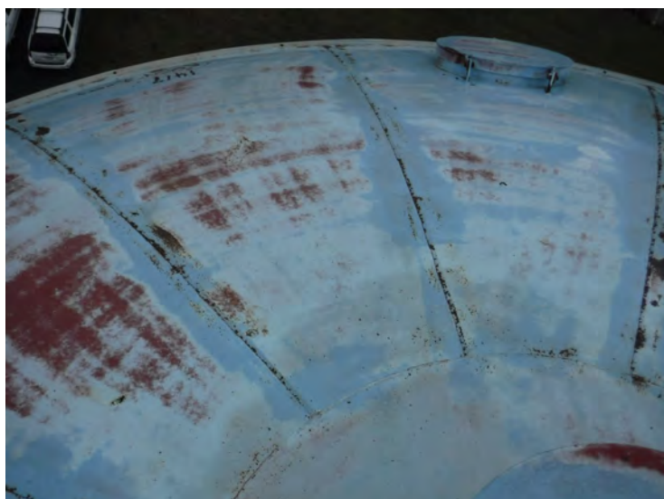
15) Primer bleedthrough and erosion throughout the roof. The secondary roof hatch appears to be in good condition.
