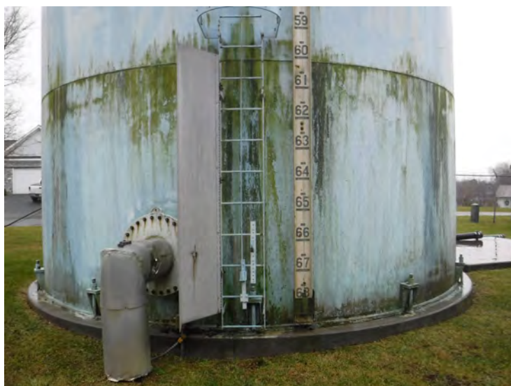
9) The vandal guard and level indicator are in good condition.
