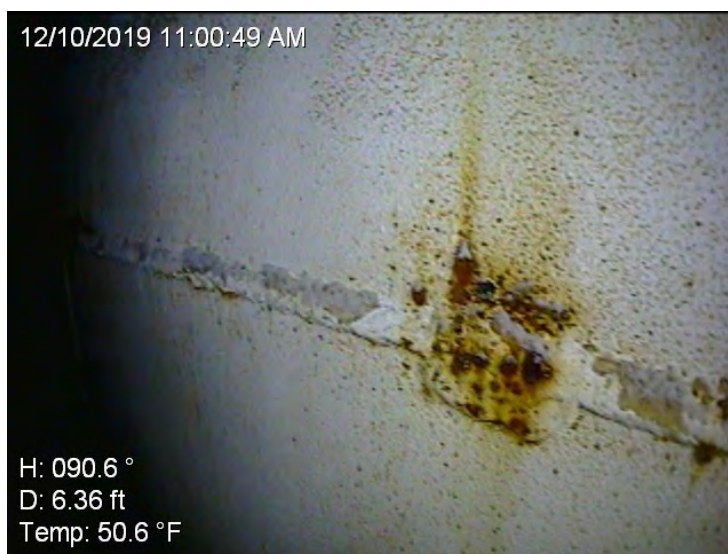
23) Spot coating failures on the sidewall weld seams.
