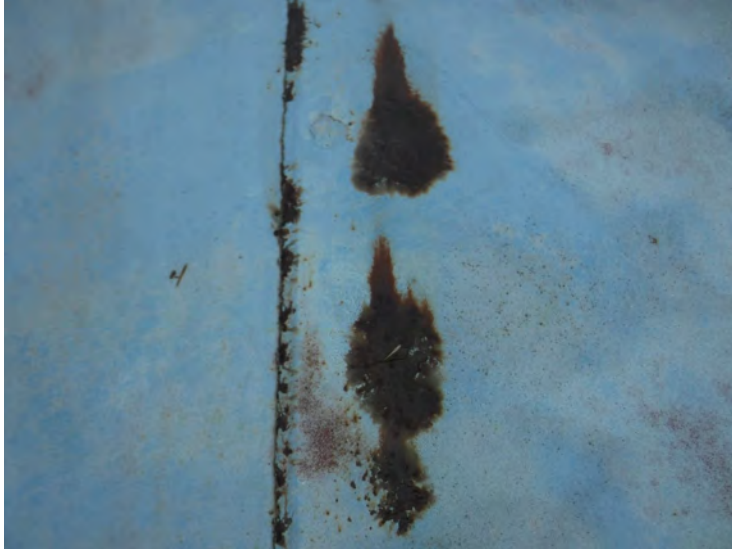
16) Spot coating failures on the roof.
