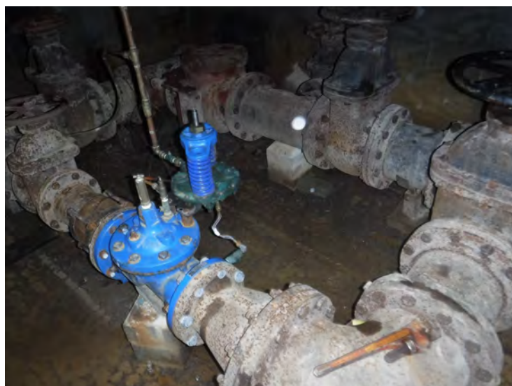
36) There are extensive coating failures on the pit piping.
