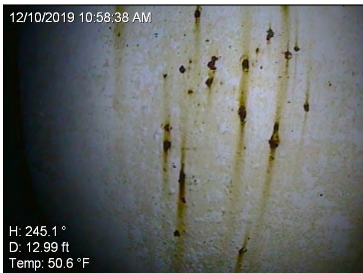
24) Spot coating failures on the sidewall.
