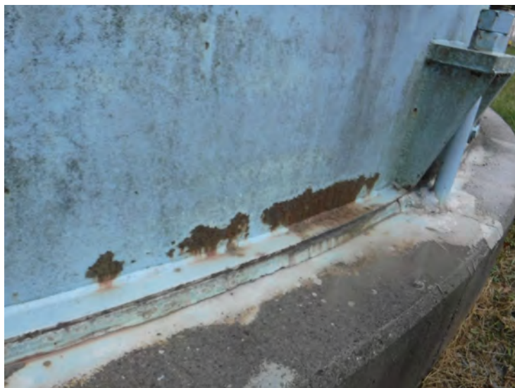
12) Spot coating failures on the lower sidewall.
