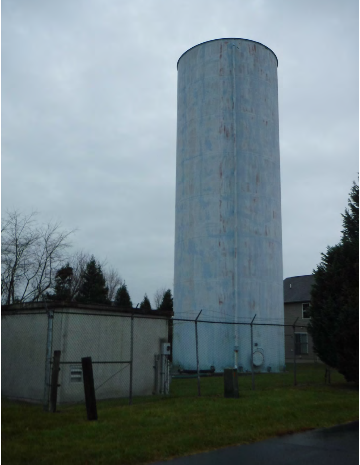
200,000 gallon standpipe (Stuckey Court) located in Martinsburg, West Virginia.
