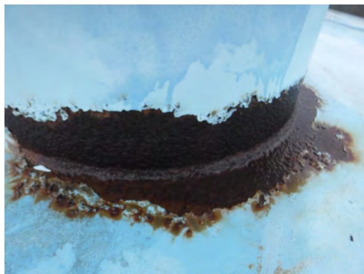
18) Coating failures on the vent neck.
