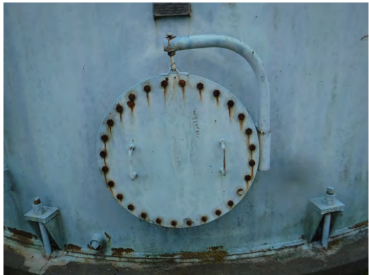
5) The sidewall manway is in good condition with minor corrosion on the bolts.
