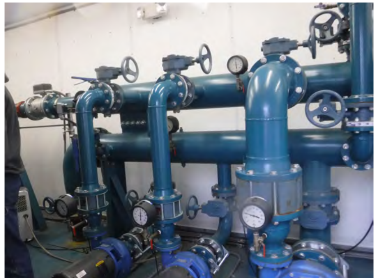
35) The coating on the piping inside the building is in good condition.
