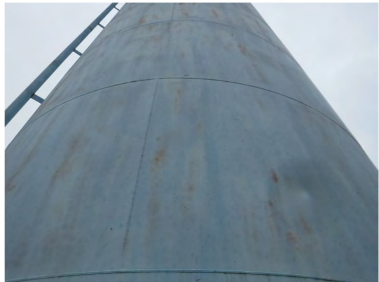
11) The sidewall coating is faded and there is erosion and rust bleedthrough throughout.
