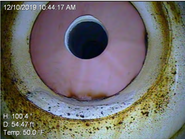
30) Spot coating failures on the second manway with fill pipe penetration.
