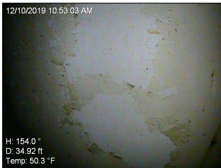
26) Topcoat delamination on the sidewall.
