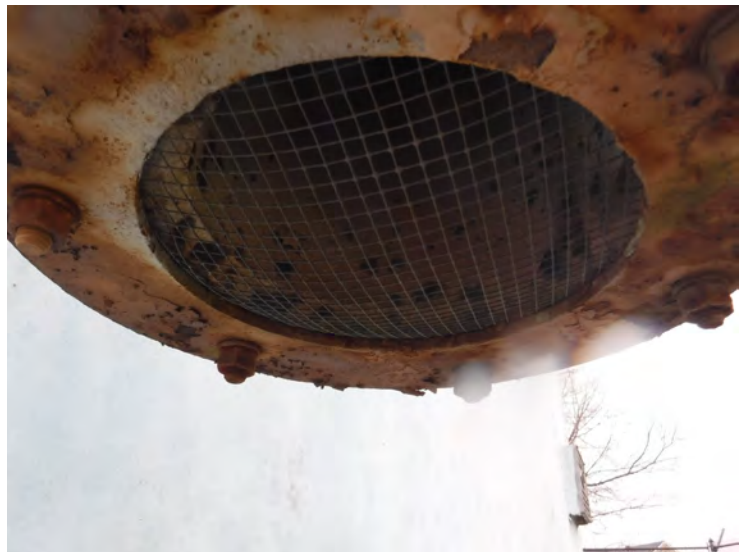
8) The overflow screen is intact but is oversized.
