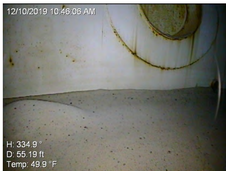
32) Sediment build-up on the floor.
