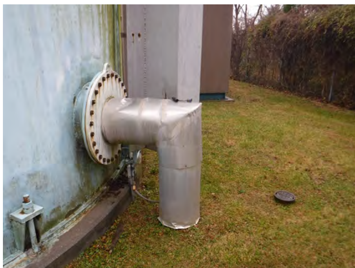
6) The fill pipe penetrates through the second sidewall manway.
