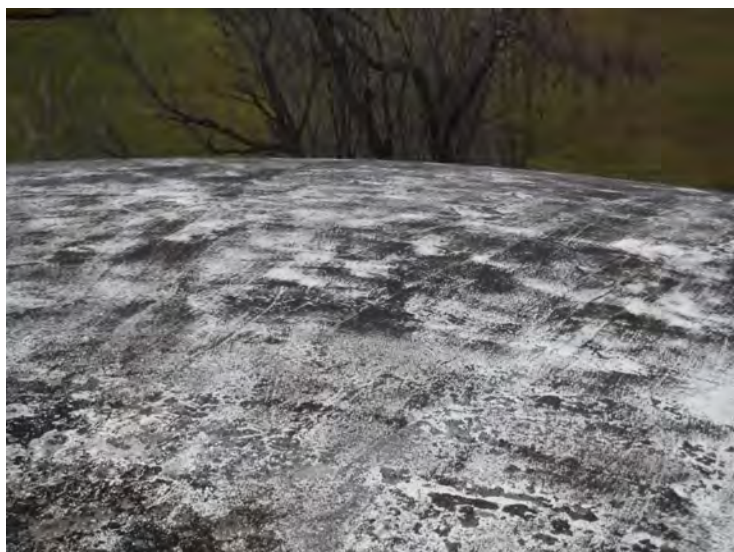
9) The roof coating is in poor condition.
