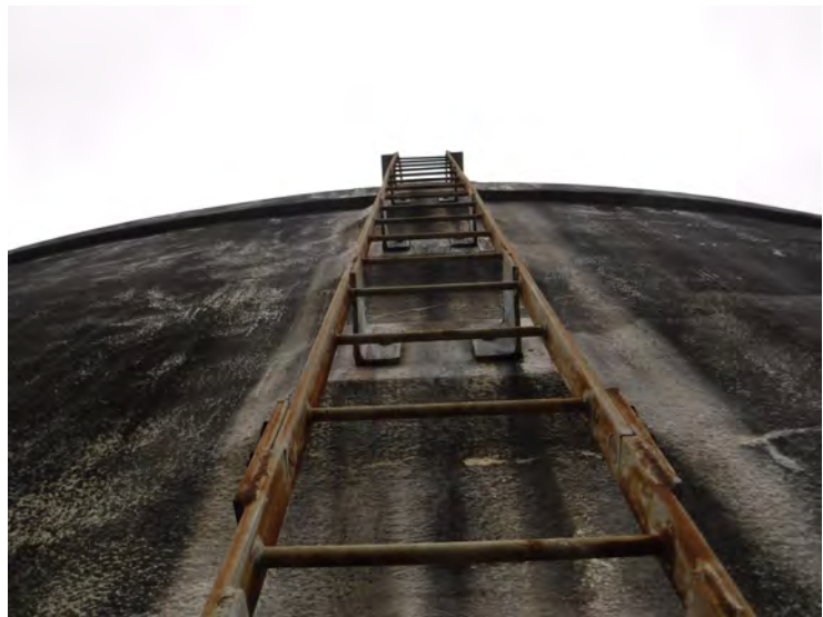
5) The exterior ladder is in good condition. The ladder is not equipped with a fall prevention device.
