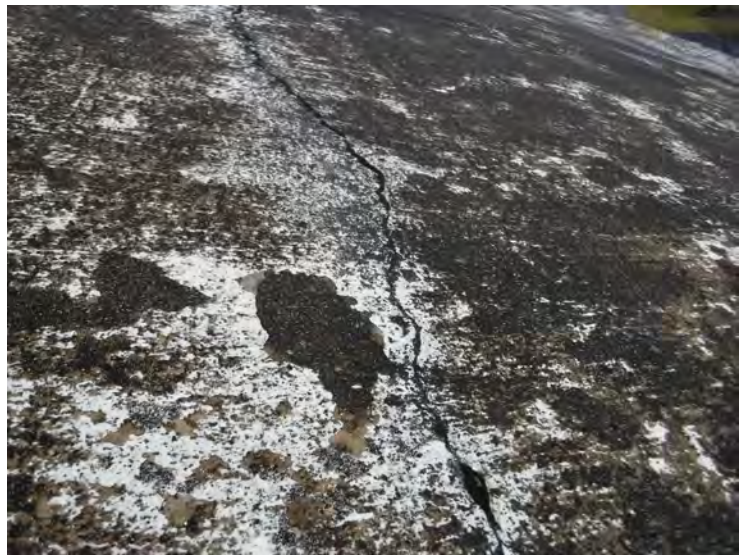
8) There is cracking on the roof.
