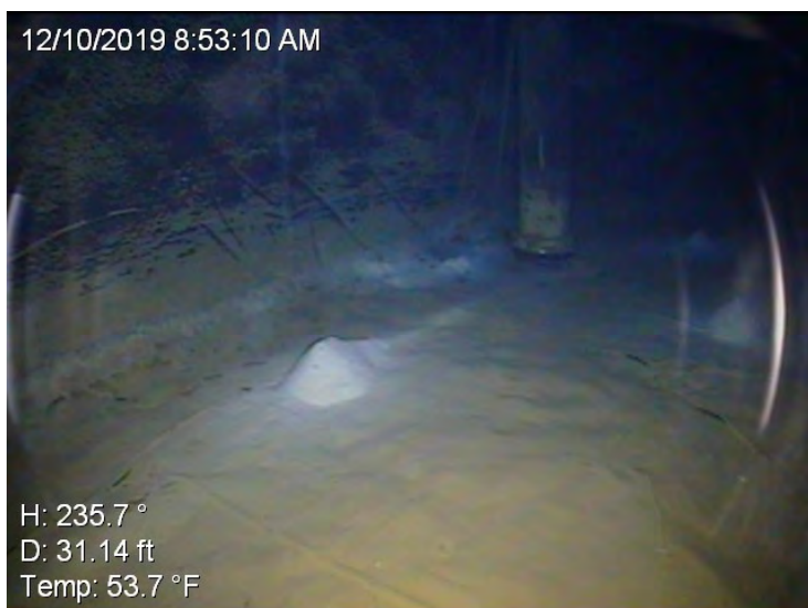
21) The floor was covered in sediment.
