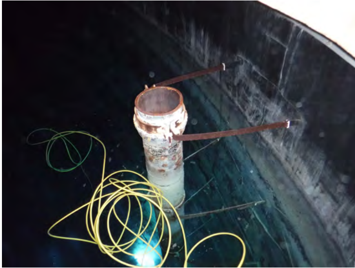
16) The overflow intake is in good condition. There is corrosion on the braces.
