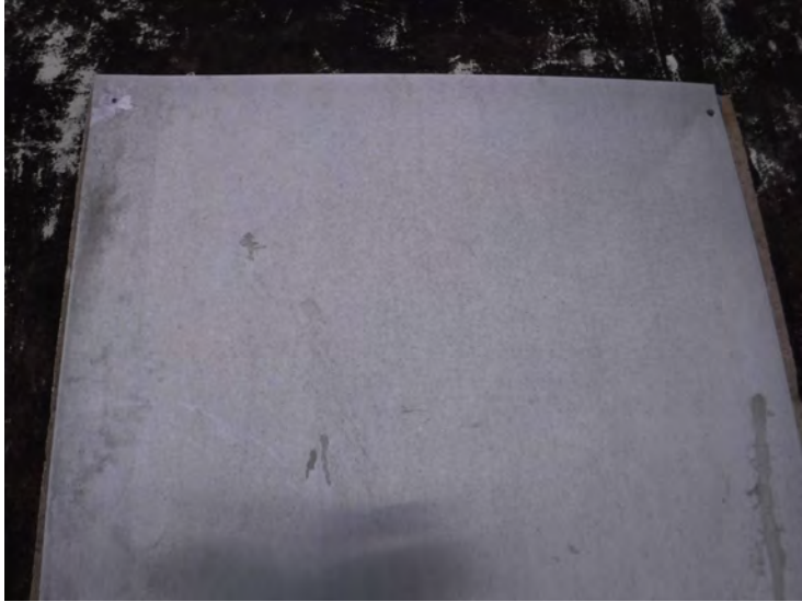
13) The roof access opening is covered with a flat piece of sheet metal.
