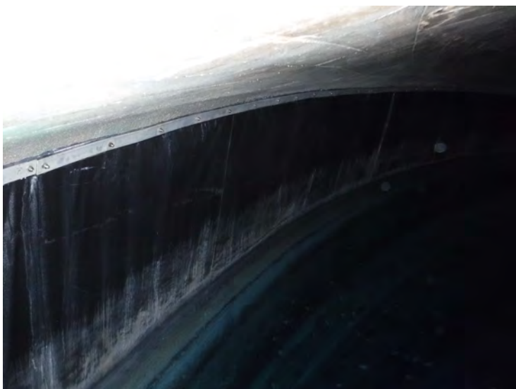
15) The sidewall is covered with a rubber membrane. The membrane is in good condition.
