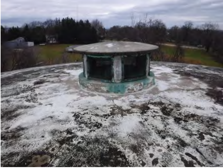
10) The roof vent is in fair condition. The vent does not have a rain shield.
