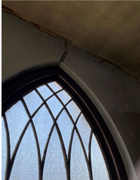
Typical crack on exterior wall
