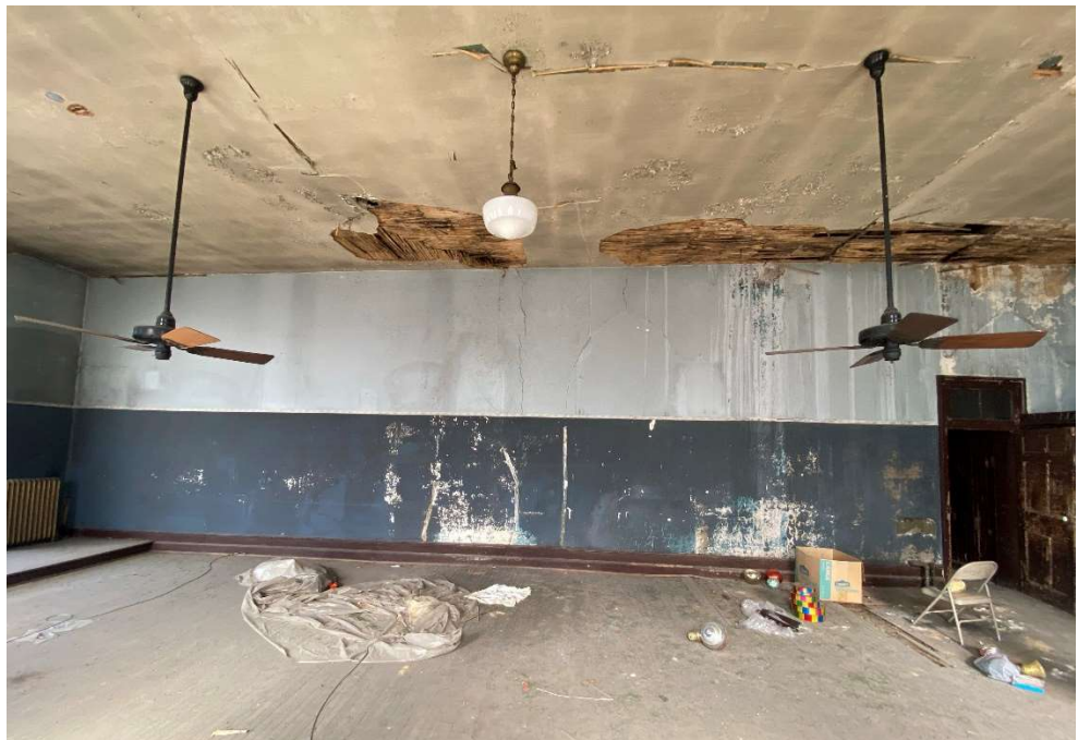
West wall of the East End Ballroom showing water damage
