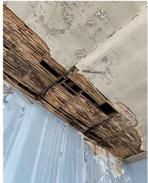
Wall and ceiling deterioration
